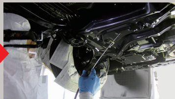
Spray "Translucent" to the hollow areas through the existing hole (approx. 0.25-0.5 l)
